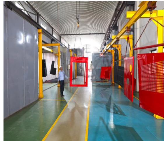
Shot Blasting Unit, Powder Coating and Liquid Paint Shop
