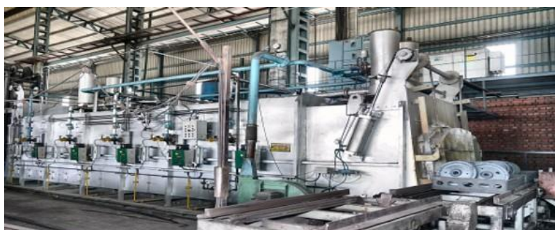
Continuous batch type heat treatment furnace
